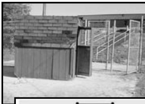
The current 8 Mile Stadium main entrance is not able to accommodate the large number of spectators on a stairway that is steep, narrow and not ADA accessible.
